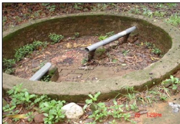
Recharging of a well in Loreto Convent School, Ranchi through roof rain water harvesting
