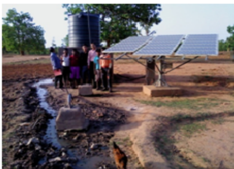
Water lifting using photovoltaic water pumps
